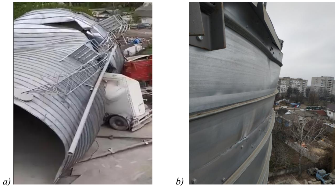
Fig. 4. Failures of spiral-fold silos: a) failure due to non-uniform foundation settlement; b) wall deformation due to incorrect operation.
